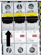
Fig.1 (Q1) Column Inverter If you close this switch, power to the inverter for movement of the carriage up/down the column is closed.
