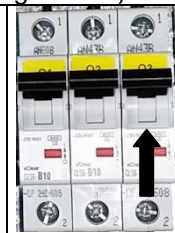
Fig.3 (Q3) Turntable Inverter If you close this turntable switch, power to the Brake (carriage's left roller) inverter is also closed.
